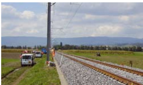
A 160 m long track was rebuilt according to the relevant standards with UIC 60 rails and concrete sleepers.
