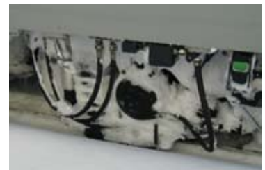
Examination of the function of the brake system and its components also under winter conditions (NSB EMU Class 72, Norway)
