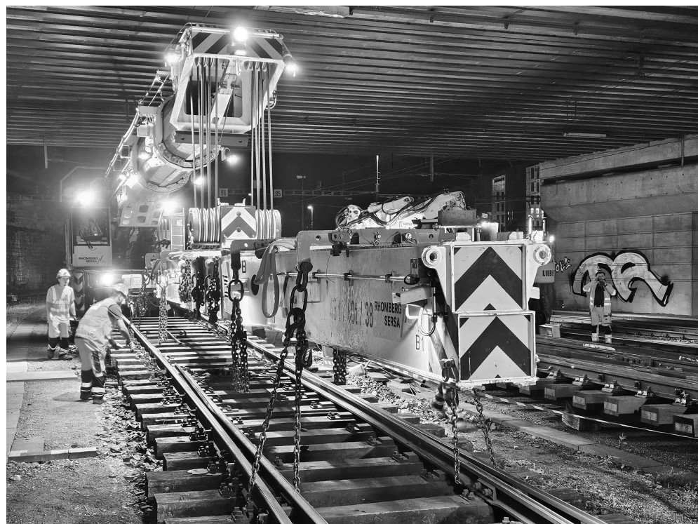
CRANE KSW 1200 BY TECHNÉ KIROW, OPERATED BY RHOMBERG SERSA (PHOTO: RHOMBERG SERSA)
