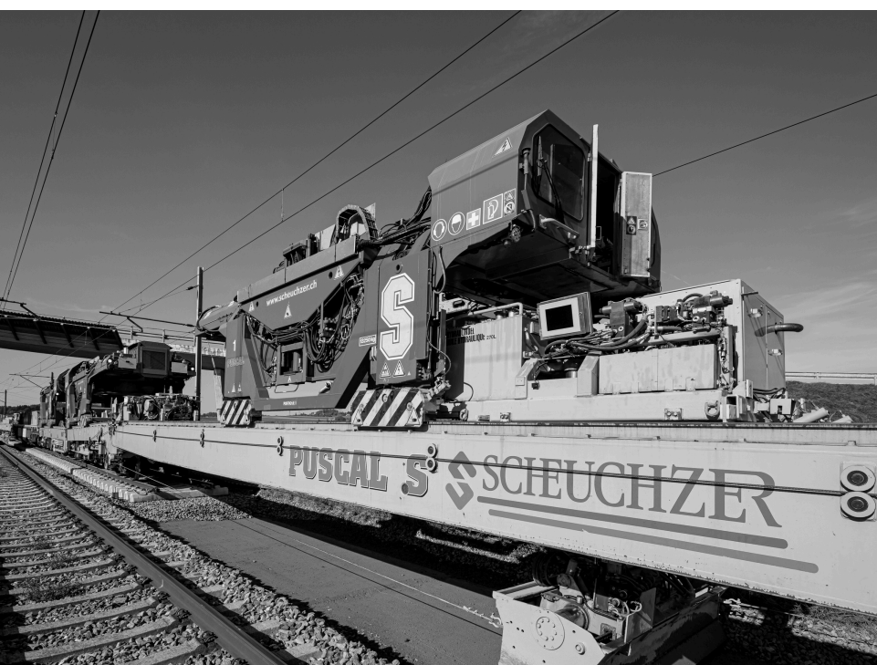
High-performance track renewal train for substructure rehabilitation in shift intervals, PUSCAL S, developed and manufactured by Scheuchzer AG and operated by Scheuchzer AG (Photo: Scheuchzer AG)
