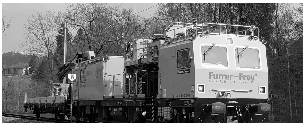
Construction train with MTW by Plasser & Theurer, operated by Furrer+Frei (Photo: Furrer+Frei)
